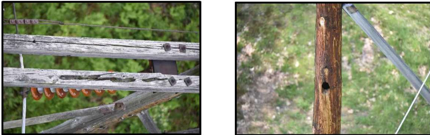
Figure 5-32 - Line 982 Asset Condition Deficiencies: cracked crossarm (left), woodpecker hole (right).
